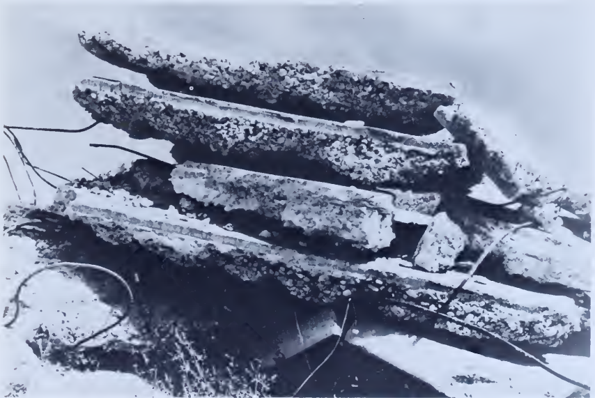
Figure 137.—A chute lining that failed because of almost complete lack of consolidation except at the surface. Most of the reinforcement steel was found to be in a useless location at the bottom of the slab. PX-D-20776.
